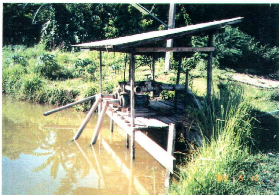
Regulating Pond and Pump for Sprinkler in Hat Dok Keo
