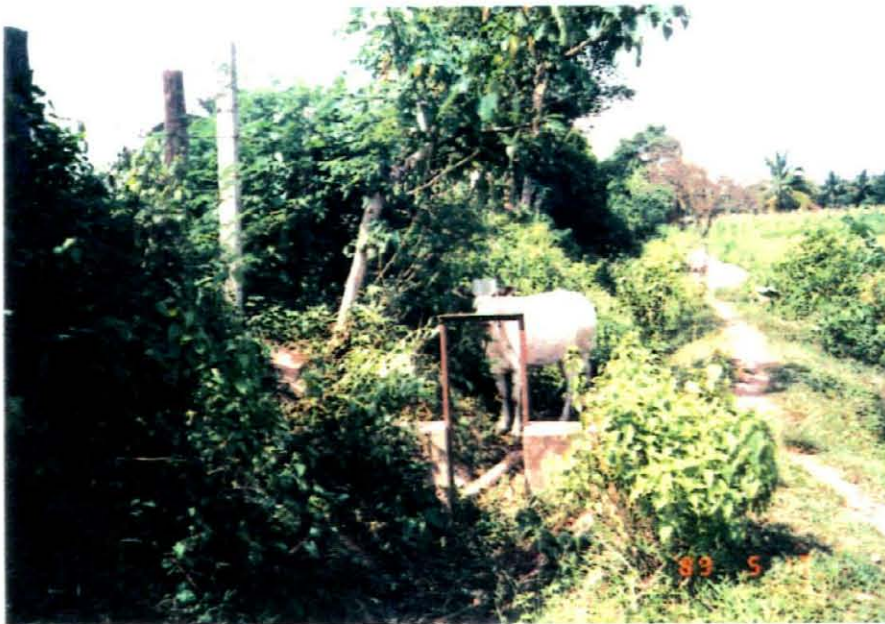
Main Canal covered with Grass and Destroyed Gate
