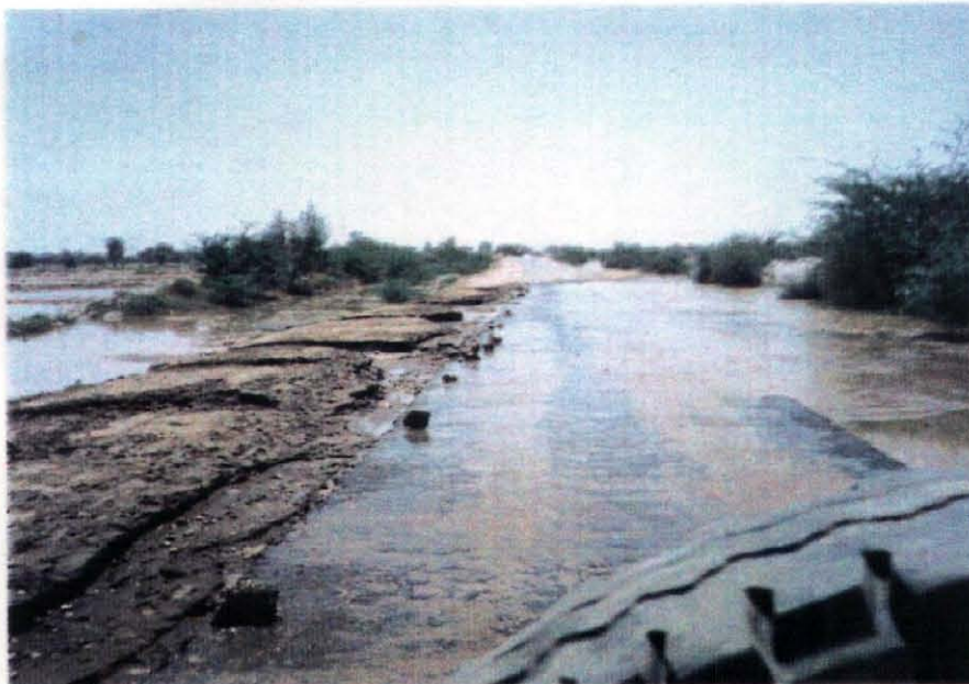
Close view of hill torrent flooding on road
