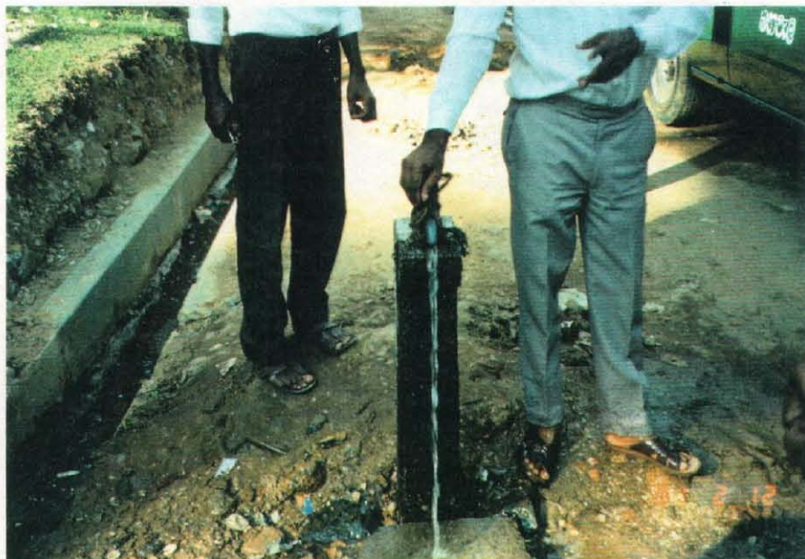
集落地区の生活用水供給用簡易水道施設 Village water supply system (water post in community area)
