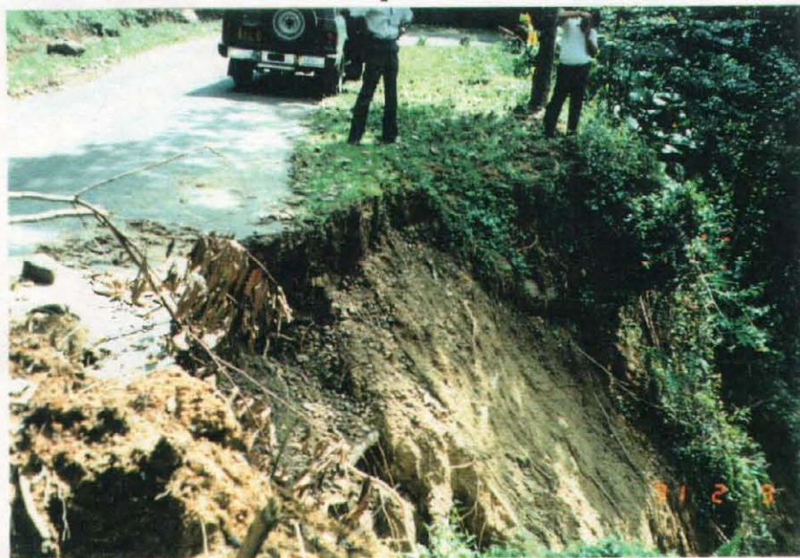
地滑り対策の必要な農道 Farm road destroyed due to land slide
