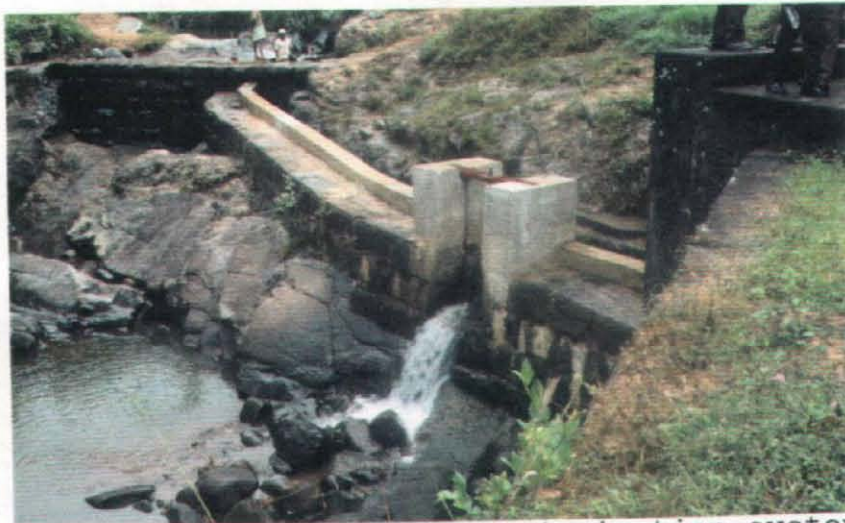
Intake facility for village irrigation system
