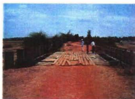
Regulator of Tumnup Lok main reservoir (to be rehabilitated)
