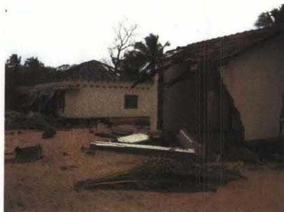
民家の被災 (アムパラ県) Collapse of houses (Ampara)
