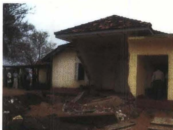
灌漑事務所の被害状況 (アンパラ県) Collapse of office building for irrigation department (Ampara)
