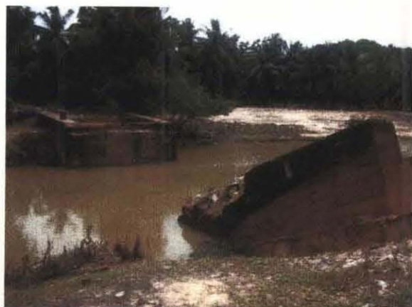
排水路橋梁の破壊 (アンパラ県) Damaged bridge over drainage canal (Ampara)
