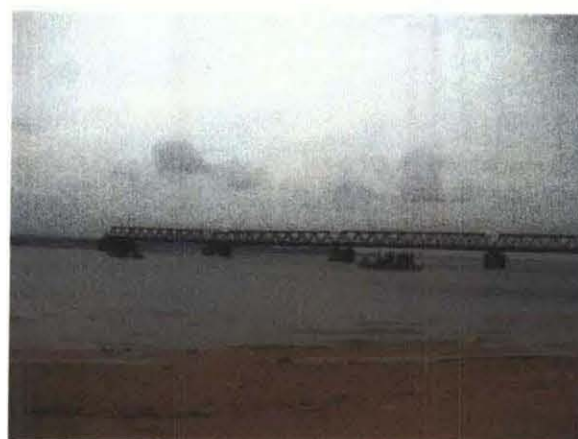
橋梁の倒壊 (アムパラ県) Damage of Bridge (Ampara)
