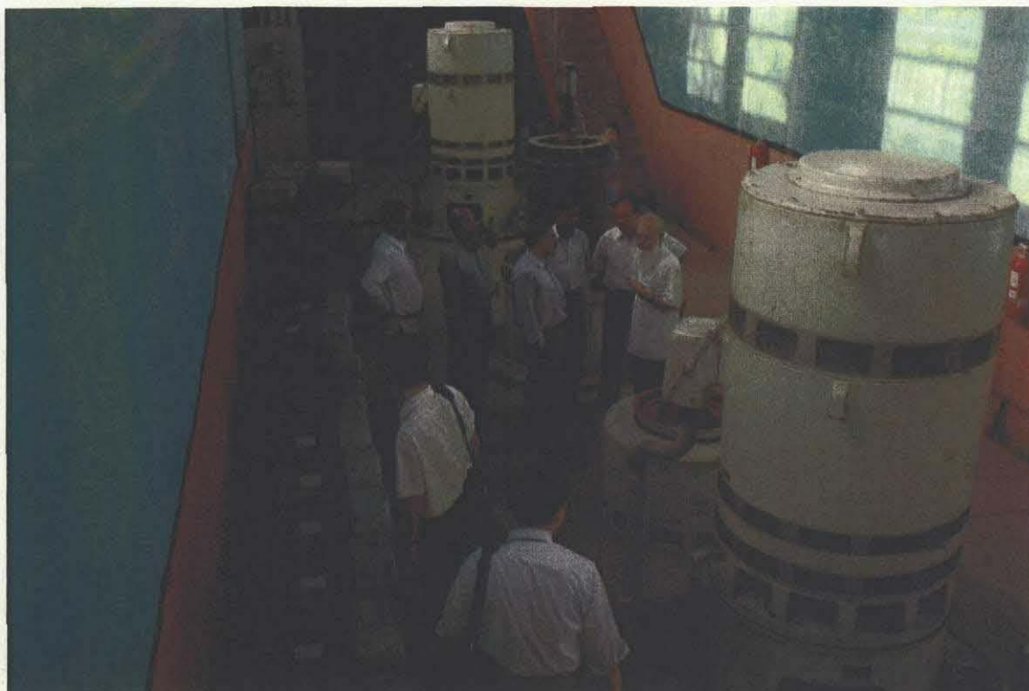
DND Pump House
